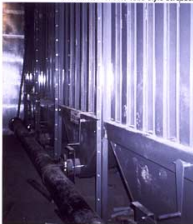
Partial view of DAS Tube-Style Scrubber
