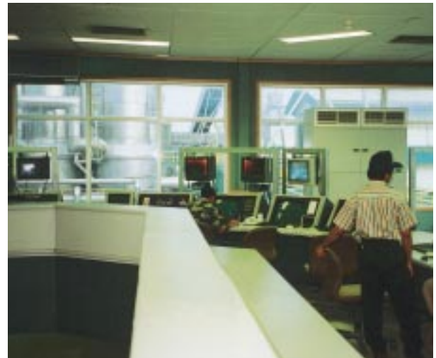
Main Control Room
